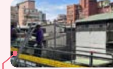
The construction frame is constructed using the handrail first frame construction method
