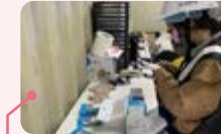
Occupational nurses randomly check the first aid kit on the construction site and confirm the medicine and date
