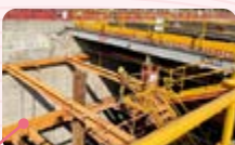
Set up safety equipment for getting on and off in the construction work area
