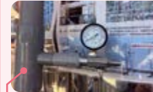
Vehicle washing station set up with flow control valve
