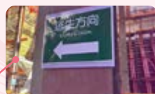
Appropriate and sufficient occupational safety publicity and safety signs
