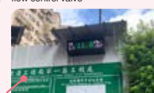
Install PM2.5 detection equipment at the entrance and exit of the construction site
