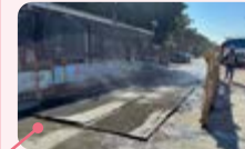
Set up a vehicle washing station and a sedimentation tank at the entrance and exit of the construction site
